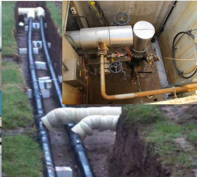
Geothermal district heating Riehen
